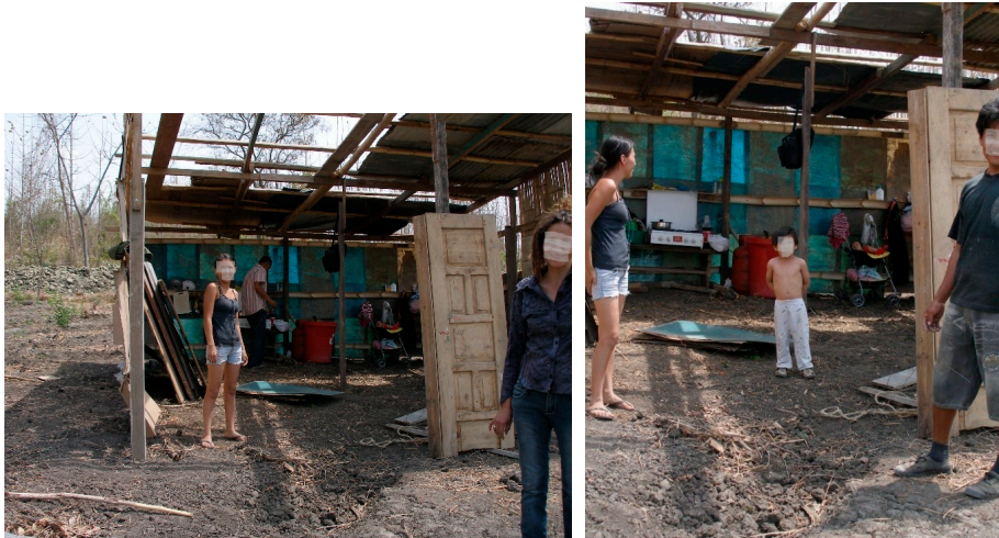
Figure 5. First day of site occupation by a new family. Construction of the new home.
