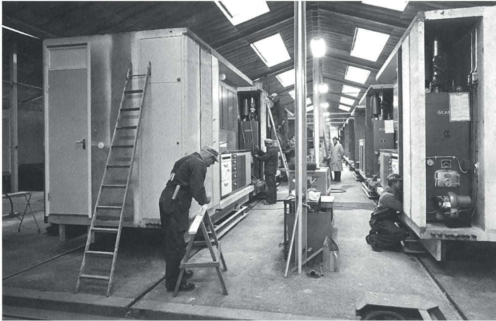
Figure 5 Factory production of volume elements including a complete kitchen, bathroom and service installations, around 1960 (Marmstål and Nordberg, 1992).
