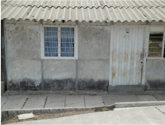
Figure 8. Second housing typology where the construction system is precast concrete panels and light metal profiles which is not suitable for incremental growth and self-construction of a second storey. Photo: Ivette Arroyo, 2009
