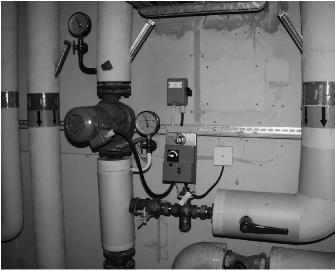
Figure 5. The control valve for the heating/ventilation system.
