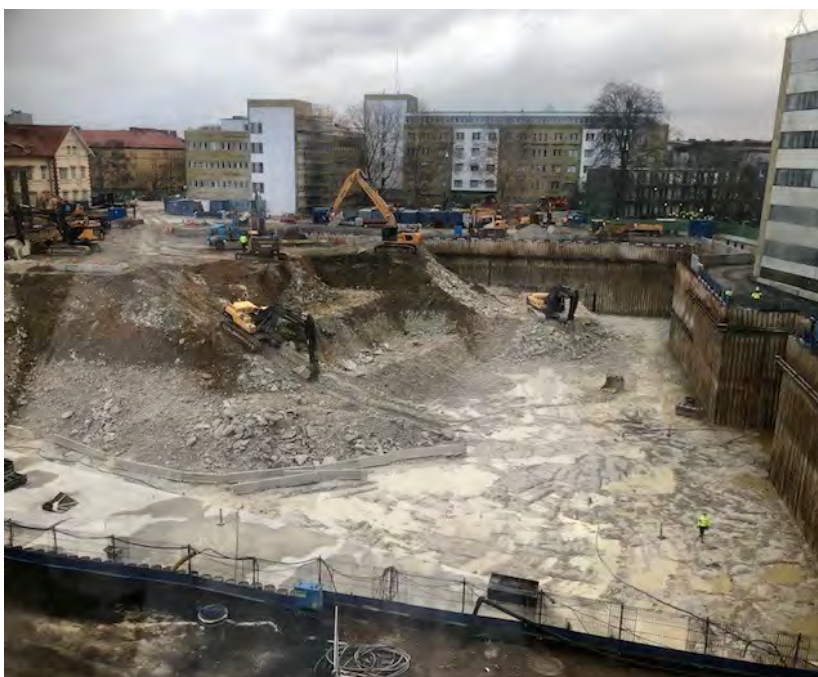
Figure 37. Excavation in preparation for new a construction at Skane University Hospital, Malmö.
