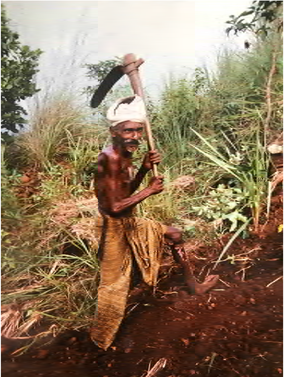
Figure 3. Construction worker digging for stones to build with, Kerala, south west India.
