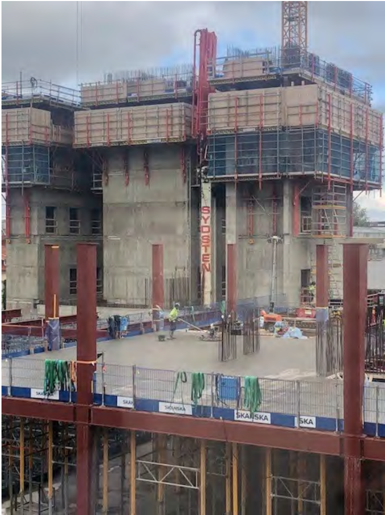
Figure 39. The new concrete building is taking form at Skane University Hospital, Malmö.
