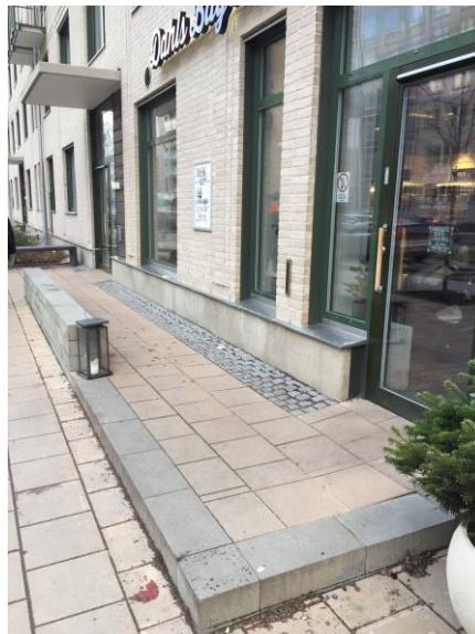
Figure 2: An entrance to a bakery in a newly built building where the level to the entrance is not even with the level of the pavement. According to regulations this difference should not be there. It could have been smoothed out by ground planning. Instead, a ramp has been built for those who cannot use the stairs.
