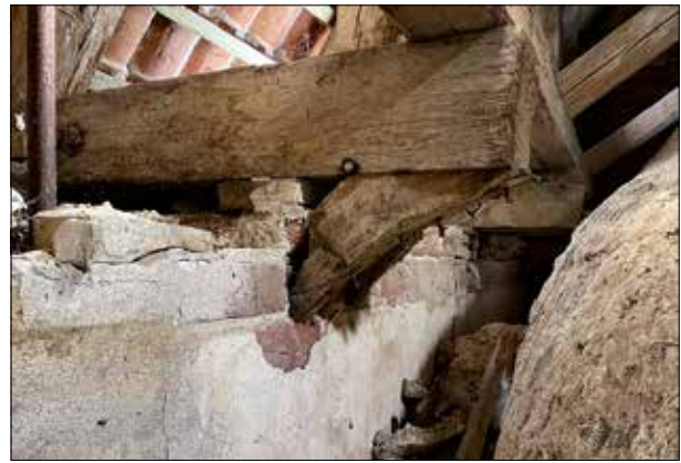
Fig. 3. Corbel under rafter foot (the original tie beam) with nails on the underside. Photo: A.C. Christensen 2023.
