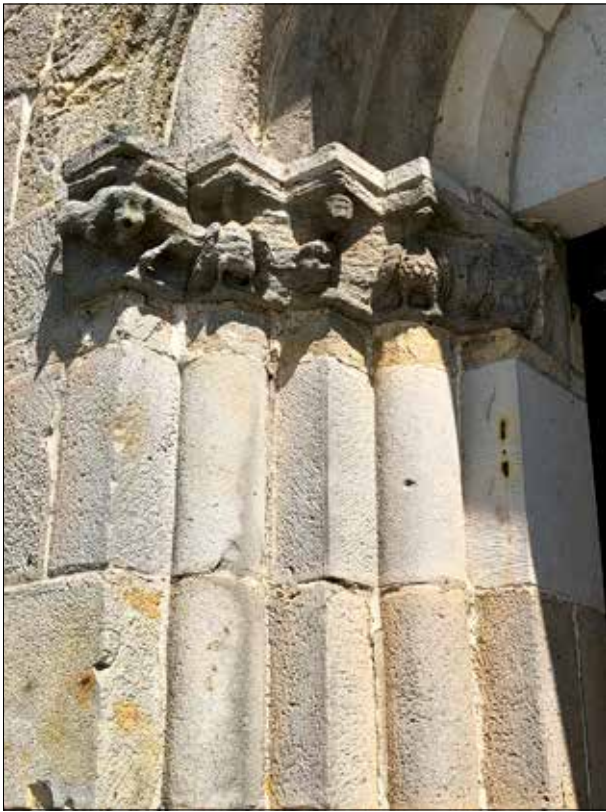
Fig. 3. In all stages of construction, the church was built of sandstone of different qualities. The picture shows the northern row of capitals at the western portal, made of a very 'clayey' sandstone and almost completely destroyed. It is surrounded by many different qualities of sandstone from the 12th century to modern times. Photo: Chatarina Ödman 2020.
