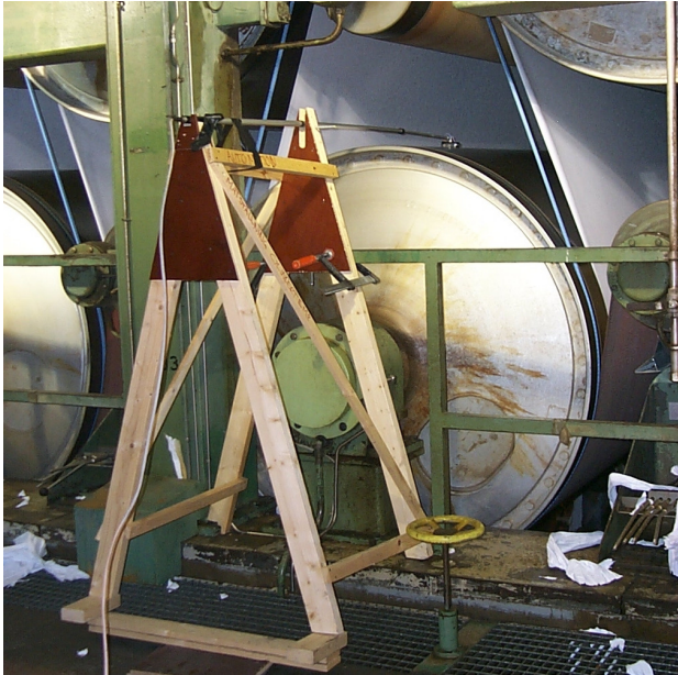
Figure 5.6 Steam cylinder temperature measuring
