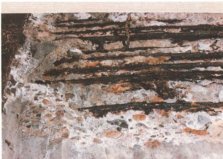
Photo 39. Corrosion of reinforcement in a traffic facility called Slussen in Stockholm where chlorides from road salt had initiated the corrosion process.
