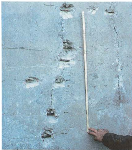
Photo 5. Photo of silo. Concrete chipped away to expose reinforcement in crack. Average centre-to-centre spacing 250 mm. Stipulated spacing 120 mm.
