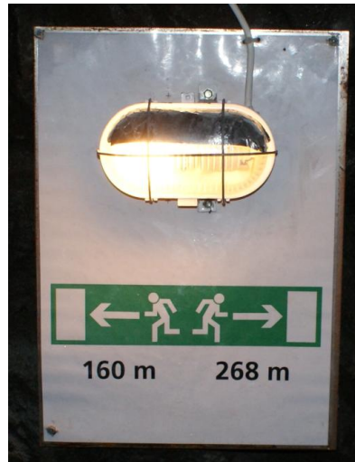
Figure 2. A picture of the emergency sign installed every eight meters inside the tunnel.
