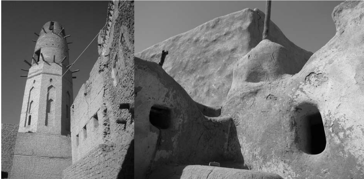
A mosque minaret that reach up to 20 meters high constructed from mud bricks.
