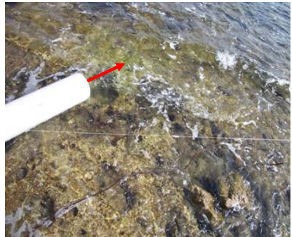
Picture 2: Brine disposal pipeline towards the sea
