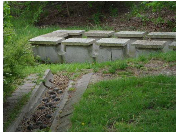
Dry canals are quickly viewed as dirty and dull by residents in the area. Image by Johanna Sörensen
