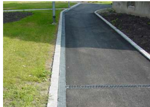
Image 8. During stage two, which developed the northern section, the open gutters were replaced by latticed gutters, and the gravel with asphalt. Image by Ulf Thysell
